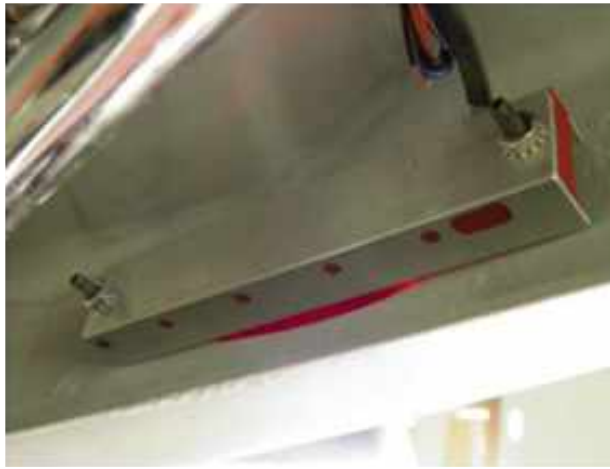
13. Ready to be wired.
